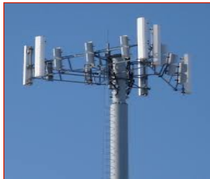
LTE BTS and small cell backhaul, enterprise “cloud” infrastructure
